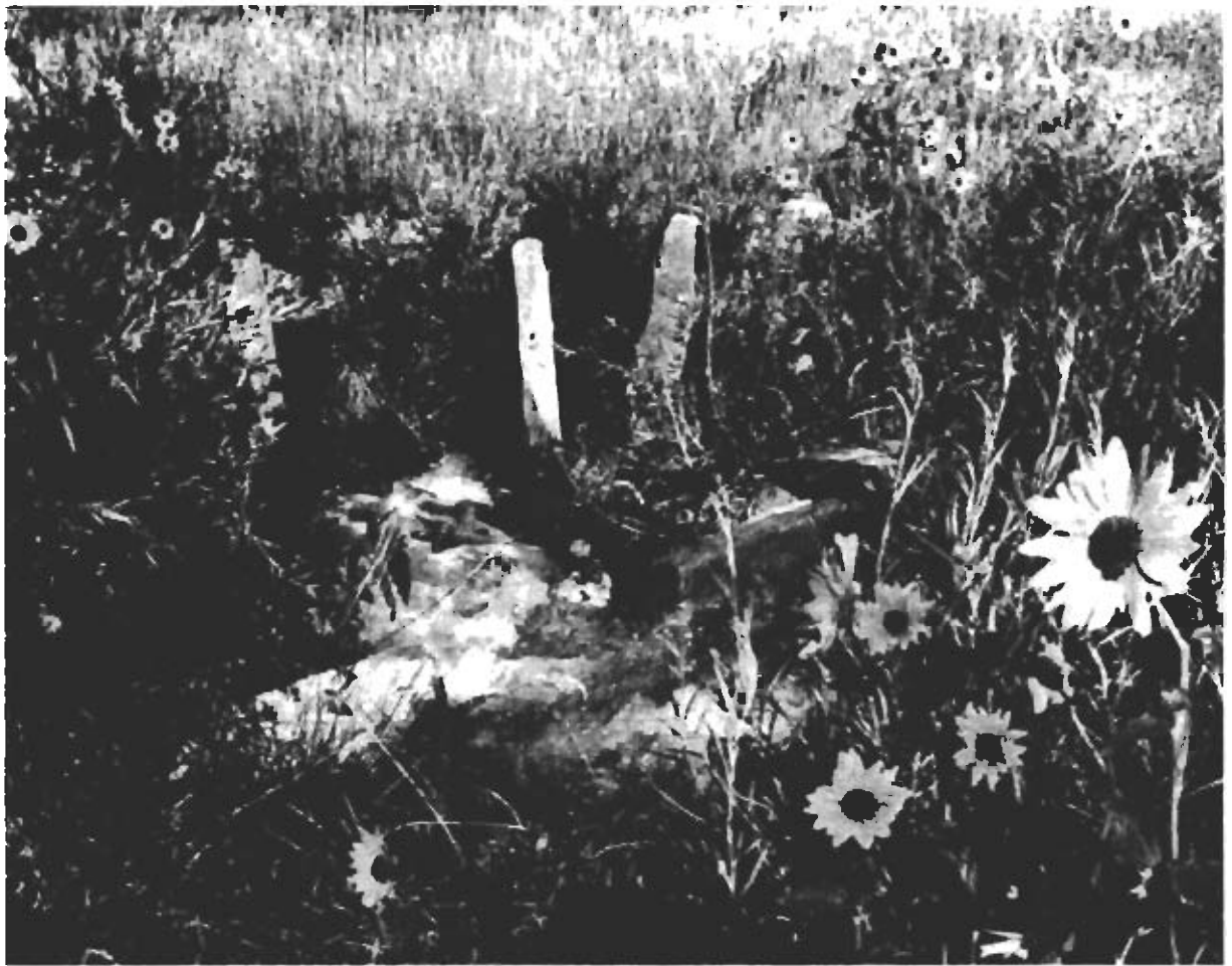
Diversion structure infested with weeds - Uinta Basin.
